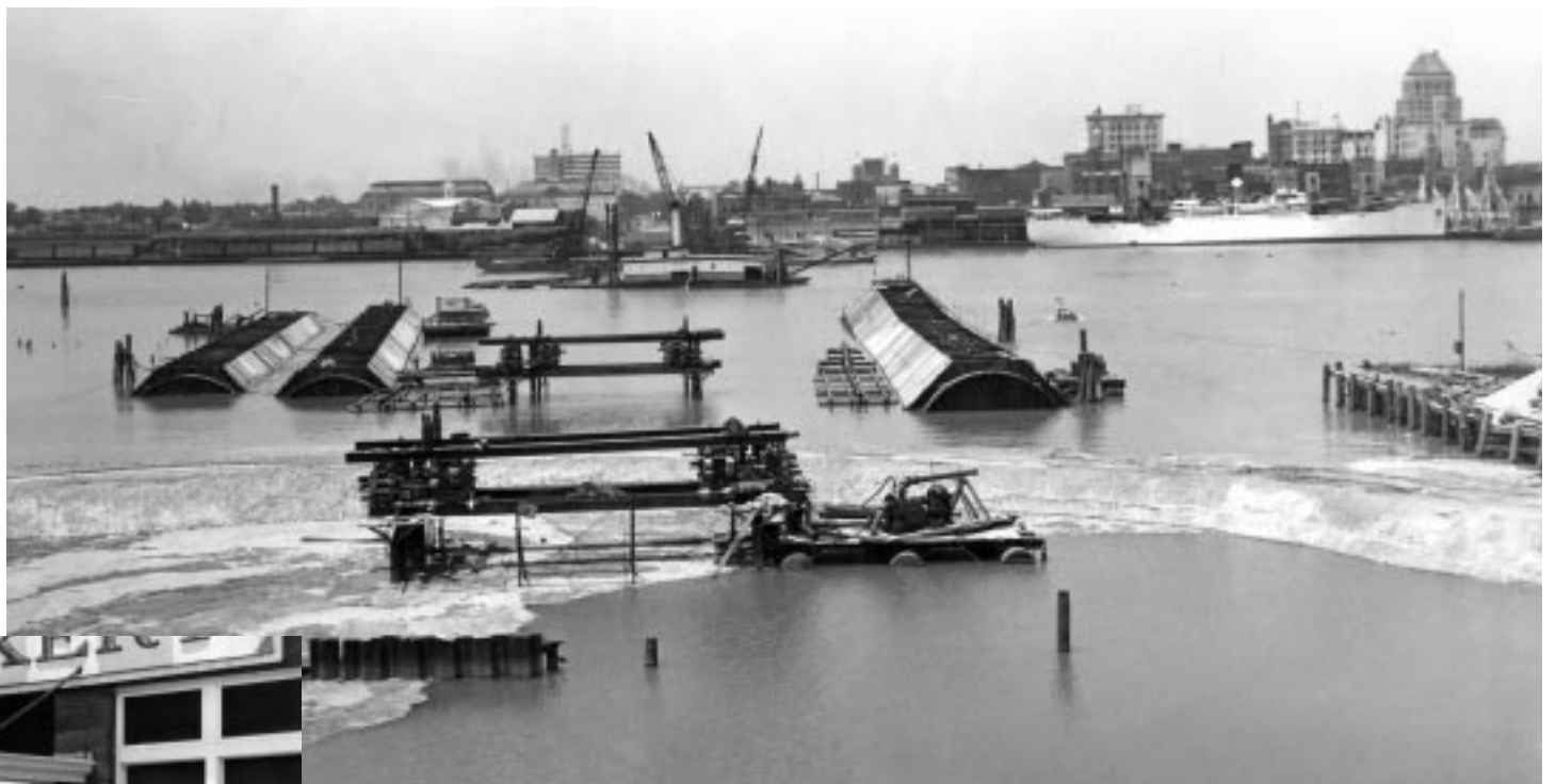
The Bankhead Tunnel under construction in June 1940. It officially opened in 1941. Erik Overbey Collection, University of South Alabama Archives
